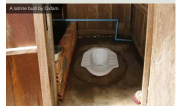
A latrine built by Oxfam.
